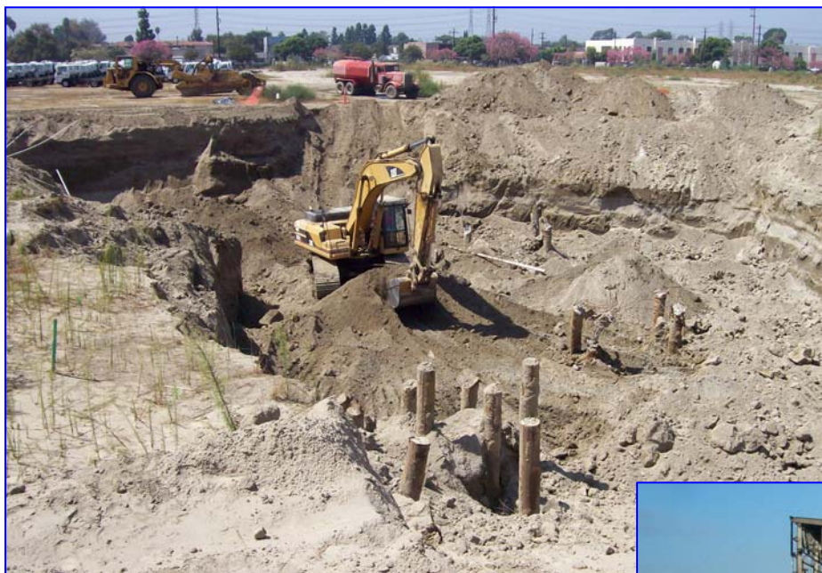
1,4-Dioxane soil excavation, structural support posts from former facility removed during excavation.
