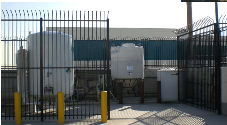
Groundwater treatment system including advanced oxidation system (HiPox) for treatment of 1,4-Dioxane impacted groundwater
