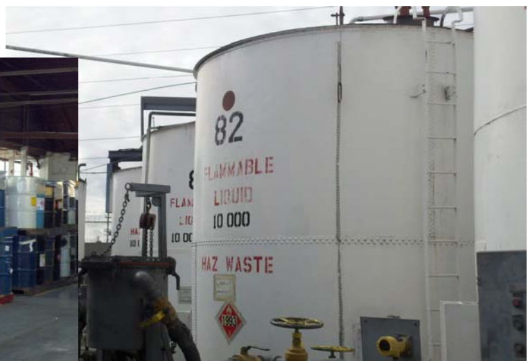
Bulk Hazardous Waste Storage Tank Farm
